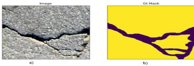
Figure 5. Crack5000 datasample. a) Image; b) groundtruth
